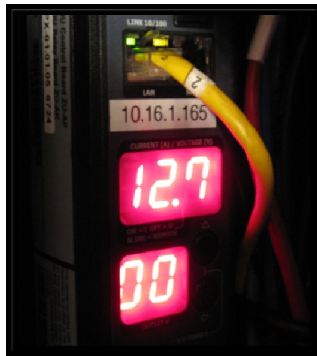
Figure 2. Raritan Dominion PX DPXS20A-30L6 deployed in J.R. Simplot's data center showing rack loads.
